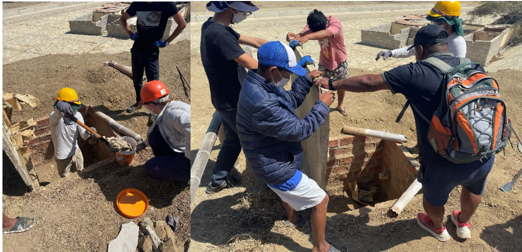
Figure 3: The team, with help from local fishermen, working to open the concrete sludge chamber to diagnose the biodigester's failure.
